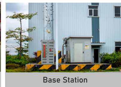
Stationary Power Generation
